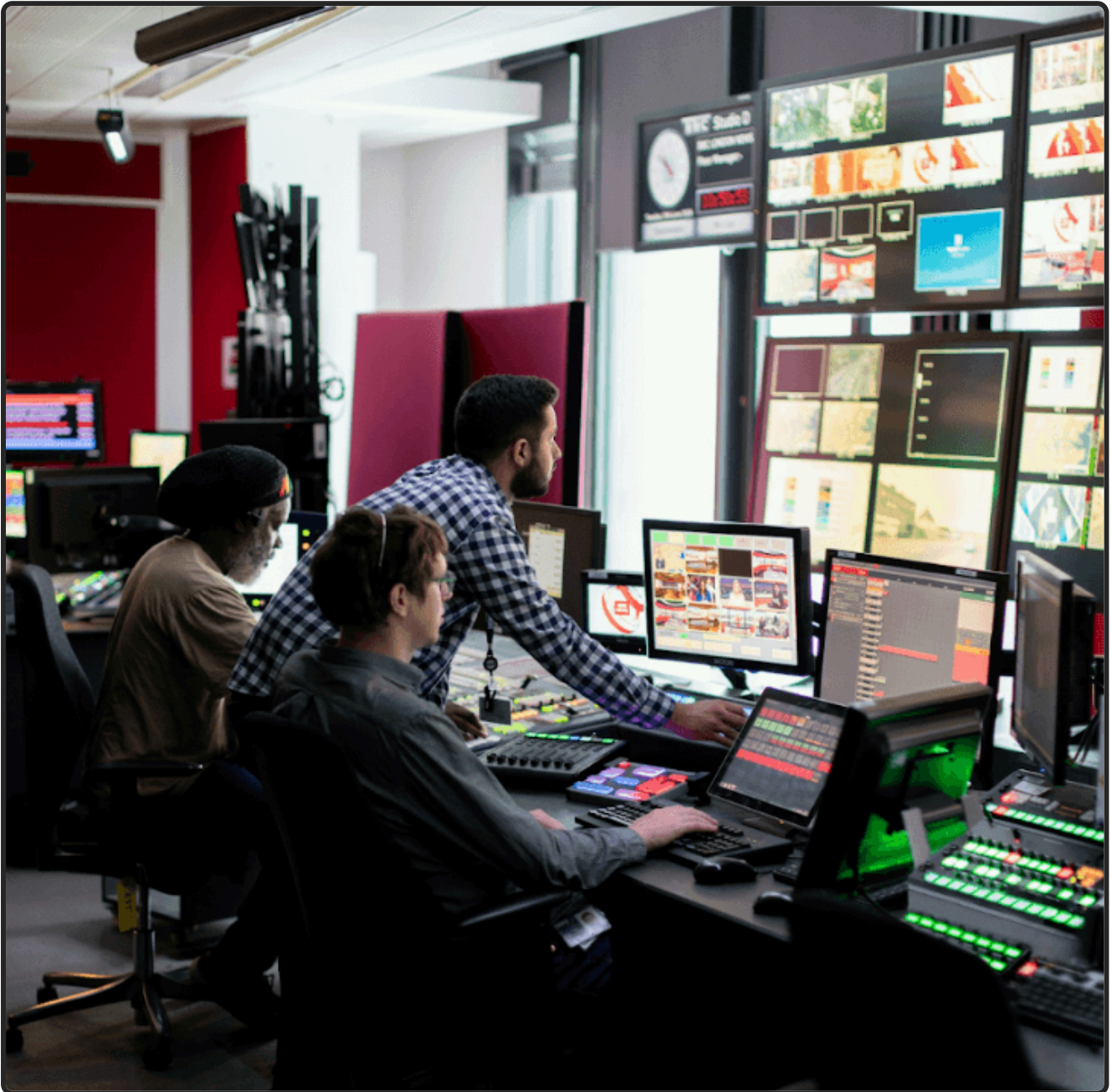
Live production control room
